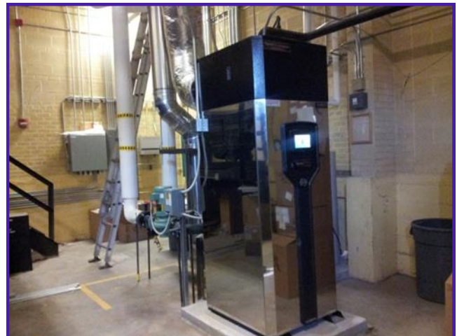
This low-NO x , high-efficiency condensing boiler was installed in 2013. Despite a 20% increase in facility square footage, the new unit used 16% less energy and saved $1,786 the first year it was operated.
