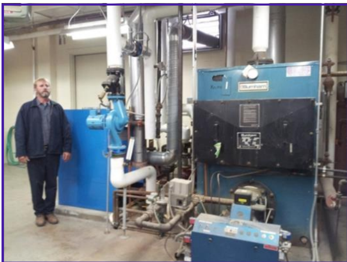
Facility manager, Mark McKenna, stands next to the new condensing hot water boiler. The old, less-efficient boiler is on the right and takes up about twice as much floor space as the new unit.
